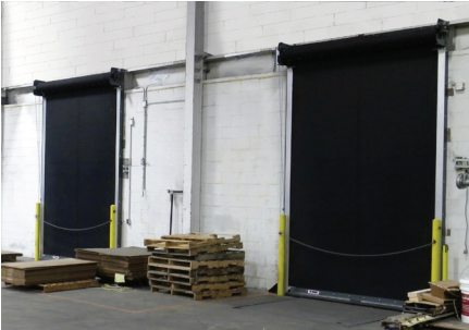
Ideal for distribution warehouse applications where accidental vehicular impact is a considerable risk.
